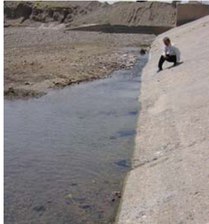
Figure 3. Water emerging from weepholes
