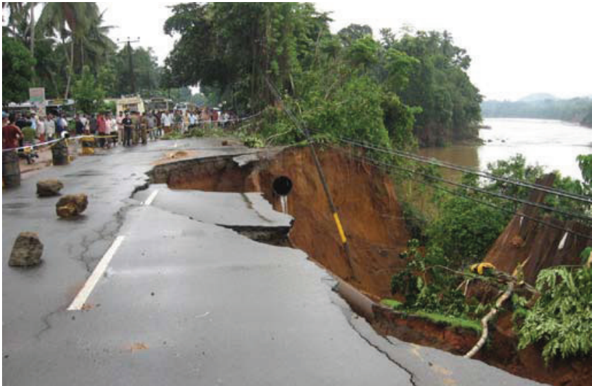
Figure 1. Kelani river bank erosion due to sand mining. A domestic water supply pipe line underneath the road got damaged and city water supply got disturbed for several days. (Photo: Badra Kamaladasa, Irrigation Department of Sri Lanka).
